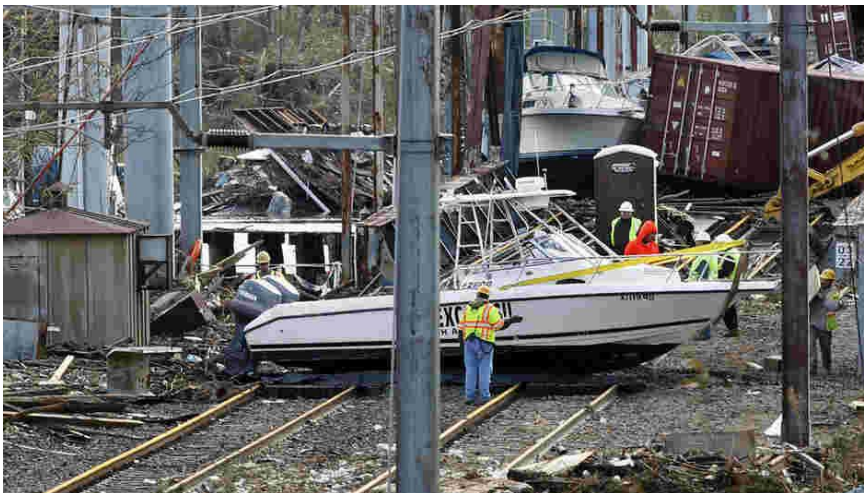
North Jersey Coast Line MP 3.1 (Morgan Drawbridge). Boats and container floated down from a Marina just North of the bridge, a bit of a unique mess!
