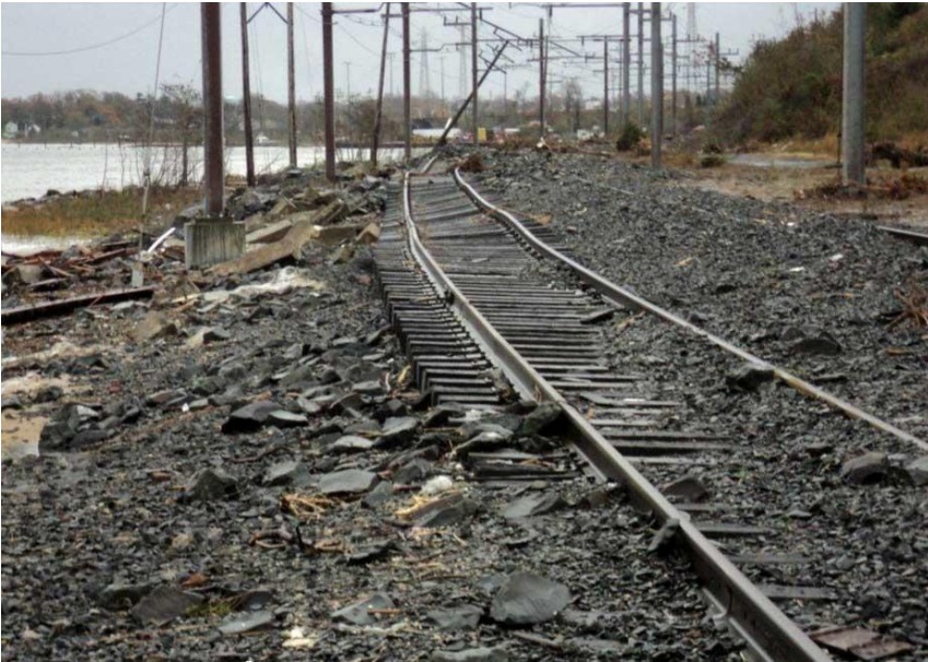
North Jersey Coast Line MP 3. Raritan Bay is to the Left. Total devastation.
