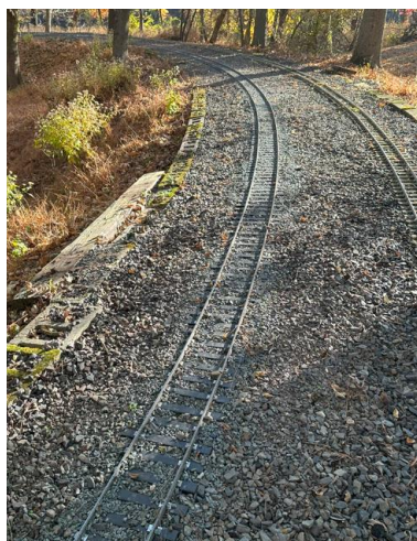
The other side of the Washout
