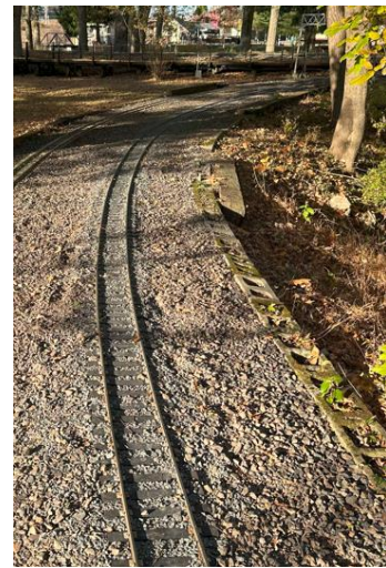
At the Washout location
